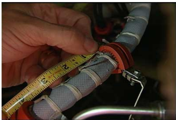
MD-80 Aux Hydraulic Pump Wiring Harness
